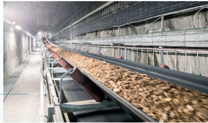
The conveyor carrying wood chips from the harbor to the boiler.
